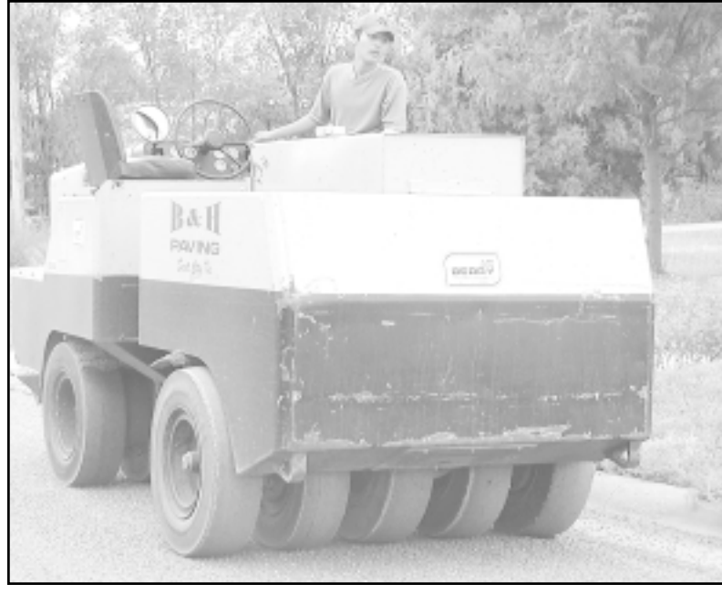
After the oil and rock are laid, a packer is driven over the road to smooth the material.
