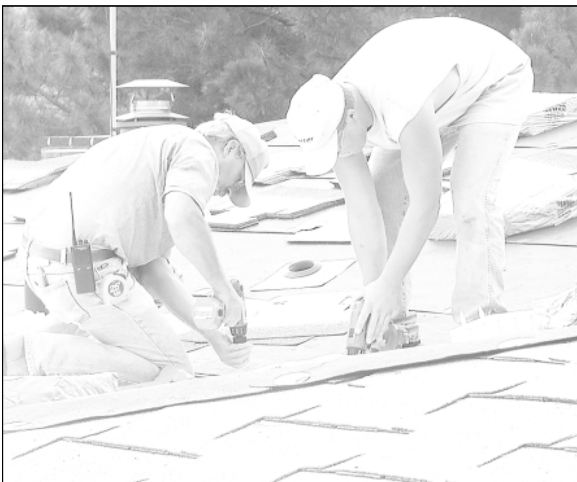
Terry Baker, owner of Terry Baker Construction, and his son Dusty were putting a new roof on a home at 605 College this morning. Photo by Doug Stephens/The Goodland Daily News
