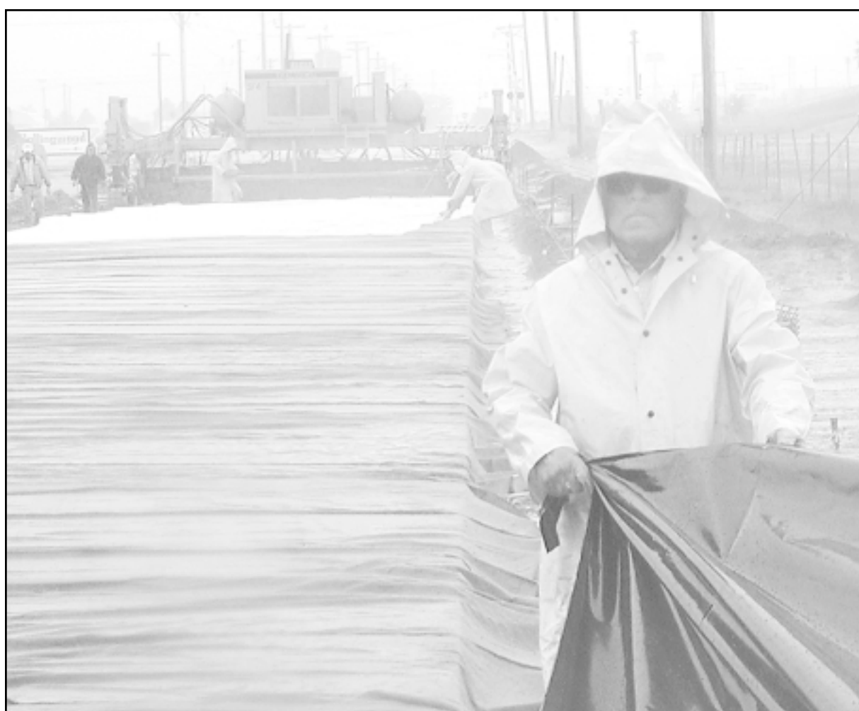
Workers from Ritchie Paving covered freshly poured cement with tarps during a thunderstorm this morning. The crew was pouring the cement on Cattletrail between 15th and 16th streets.
