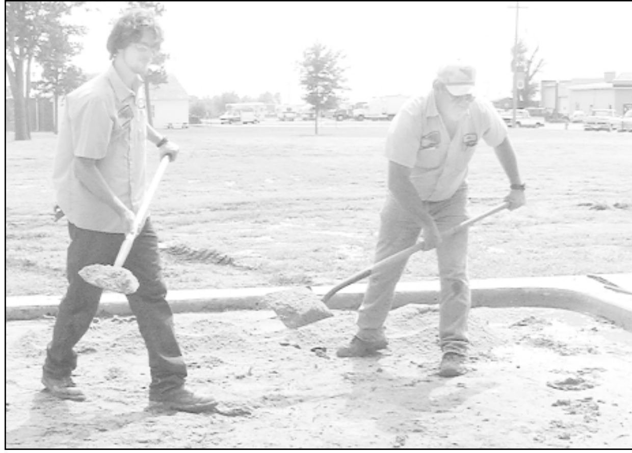
Chris Best (left) and Phil Erickson filled the old wading pool at Steever Park with sand to get it ready to pour concrete for a concert stage.
