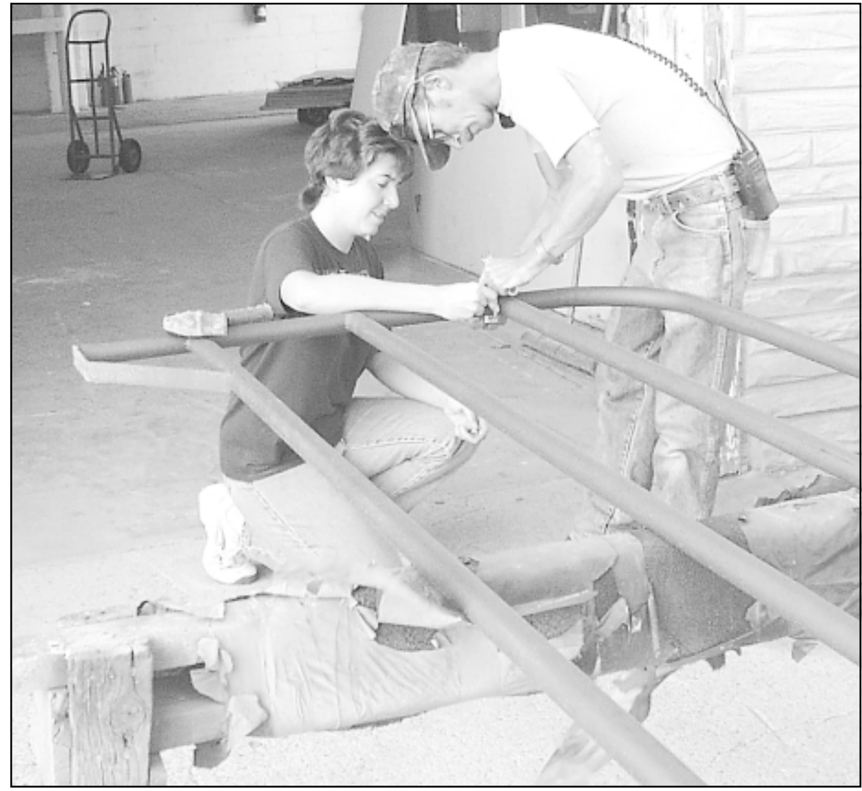
Crystal Linsner and William McKnight put clamps on one half of the metal gate being installed on the south side of the county's household hazardous waste facility at 1820 Cherry. The first collection is to be from 7 a.m. to 1 p.m. Saturday.
