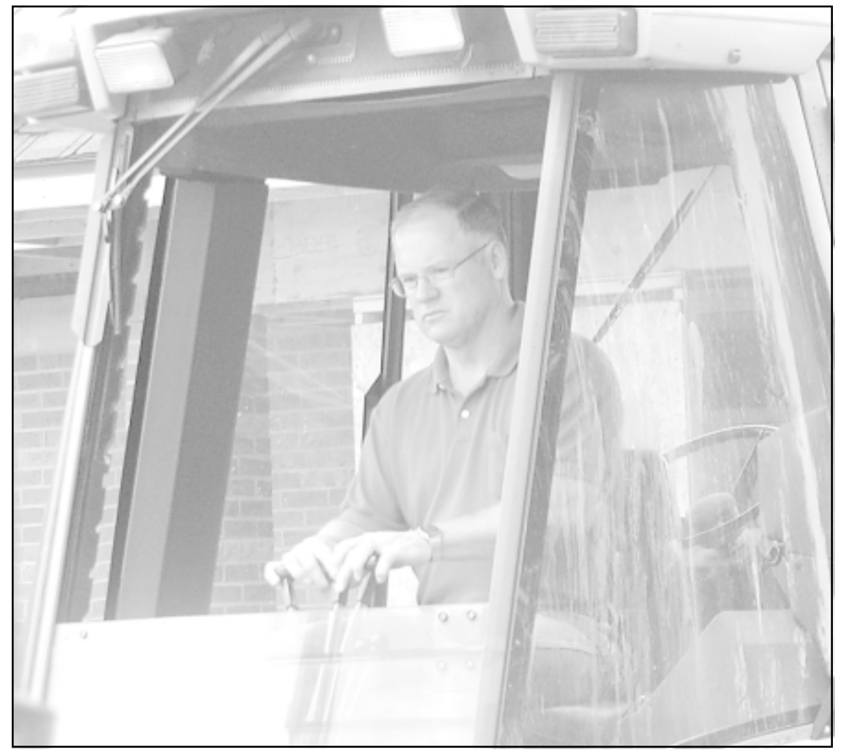
Curtis Baldwin of Rhodes Construction used a backhoe to smooth out dirt Friday in front of the new S&T Communications office. Photo by Doug Stephens/The Goodland Daily News
