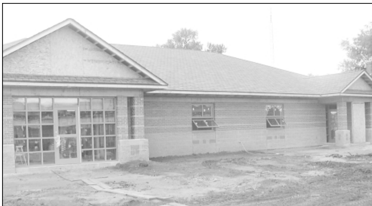
The exterior of the S&T Communications office building is mostly done. The office should be ready to open in less than two months.
