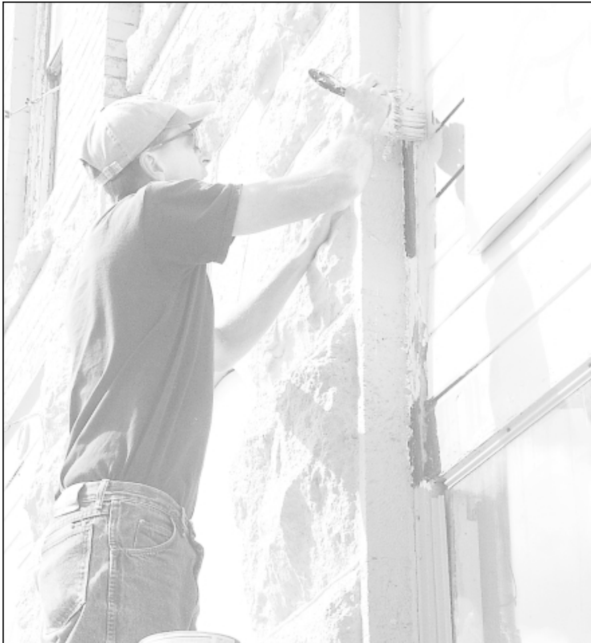
Alan Focke, a subcontractor for Stephens Construction, painted a light blue primer on the wood trim at the new Daylight Donuts shop Friday. The trim is painted dark blue, and the shop plans to open next week.
