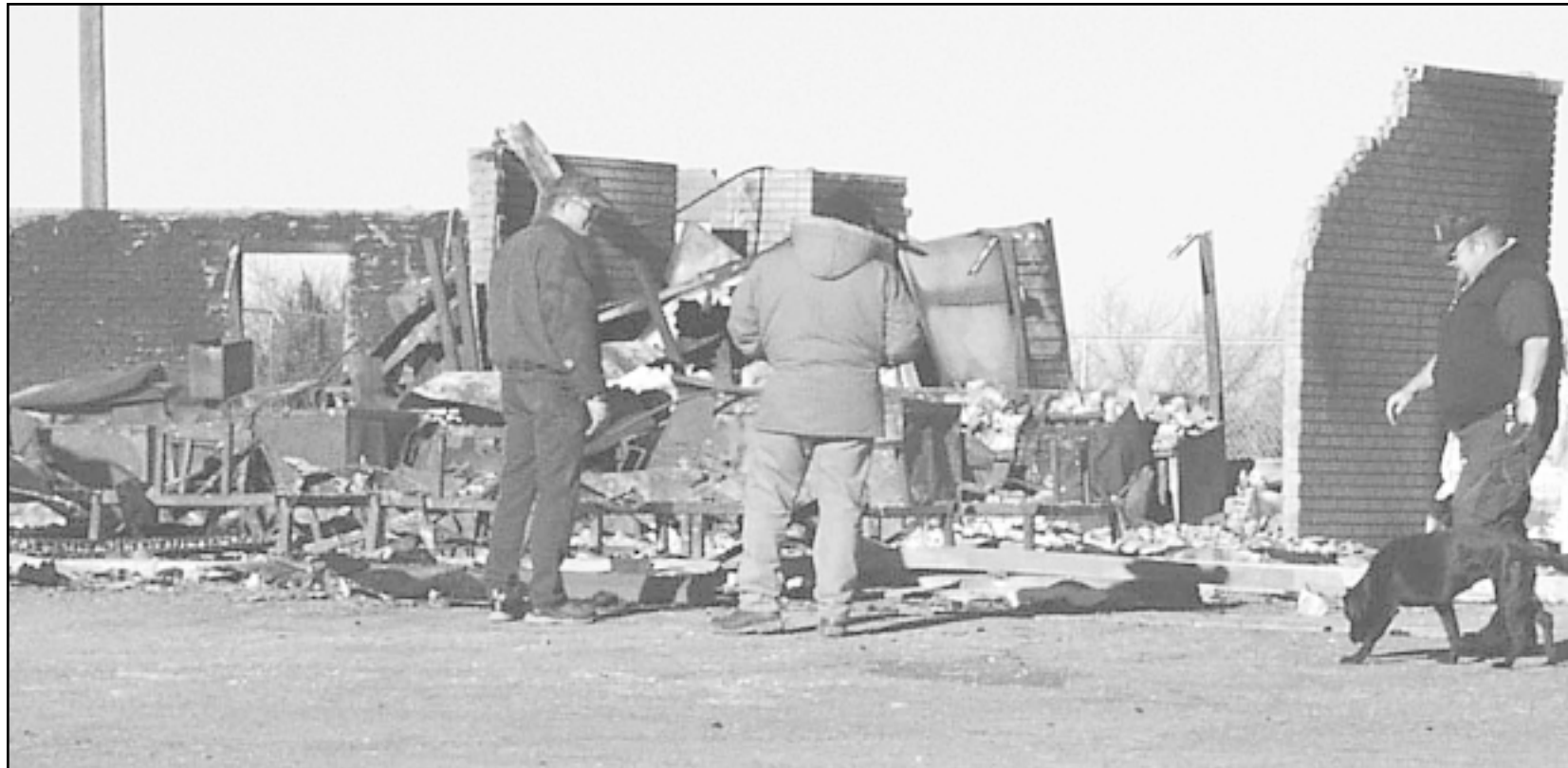
Stuckey's Restaurant, south of Brewster on I-70 about 18 miles east of Goodland, was leveled by fire on Saturday night. This morning, investigators used a dog to help find out how the fire started. The first
