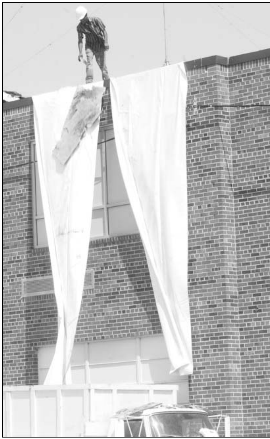
Crewmen are having to endure searing heat while refinishing the roof on the west wing of Goodland High School. The crew from Interstate Structures of Kearney, Neb., hopes to finish the entire roof by the end of the summer.
