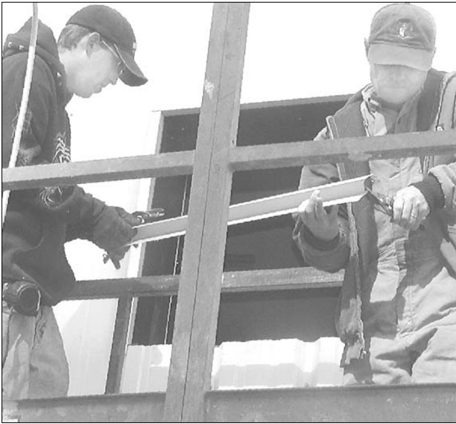
Andy Pottorf and Lowell Lambrecht, who work for Dennis Malson, owner of Malsolm Welding and Repair Service, cut the final moul-
