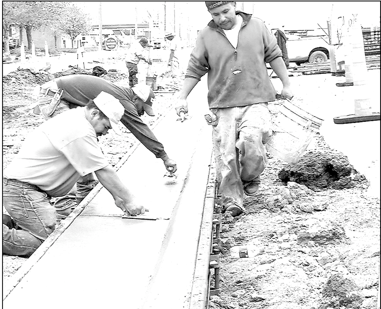
Curb and gutter work on 17th Street has nearly reached Main as workers smoothed and finished a section in front of the Antique Warehouse on Tuesday. Work continues on the intersection at Main and 17th, which is to be completed by the end of the month. To ease traffic a portion of the street near the railroad crossing has been opened to allow two-way traffic.
