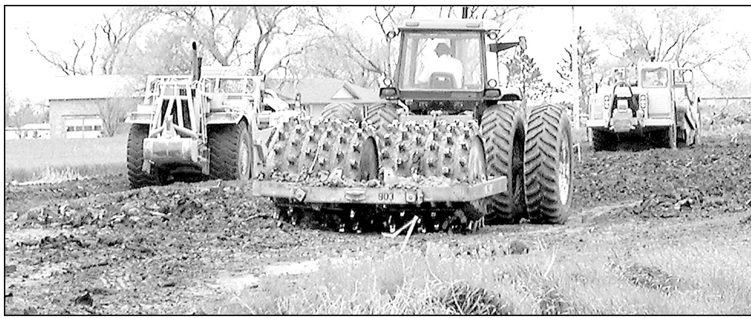
Dirt work is being completed on the shoo-fly detour south of town, and Michael Terry of the State Department of Transportation said Thursday the short detour will be the first part to be paved begin-
