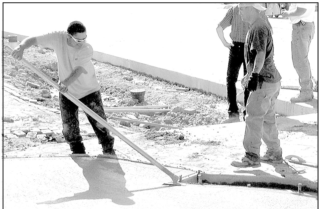
A crew from Midland Contractors of Great Bend worked on corners at 17th Street and Main on Friday. The last strip of concrete for the street was poured Monday. Traffic will be able to go east and west by the end of the week, said Darin Neufeld of Evans, Bierly, Hutchison and Associates, and turn onto Main by next Monday. The section of 17th in front of the Antique Warehouse and Hank's Cafe is open. Photo by Pat Schiefen/The Goodland Star-News
