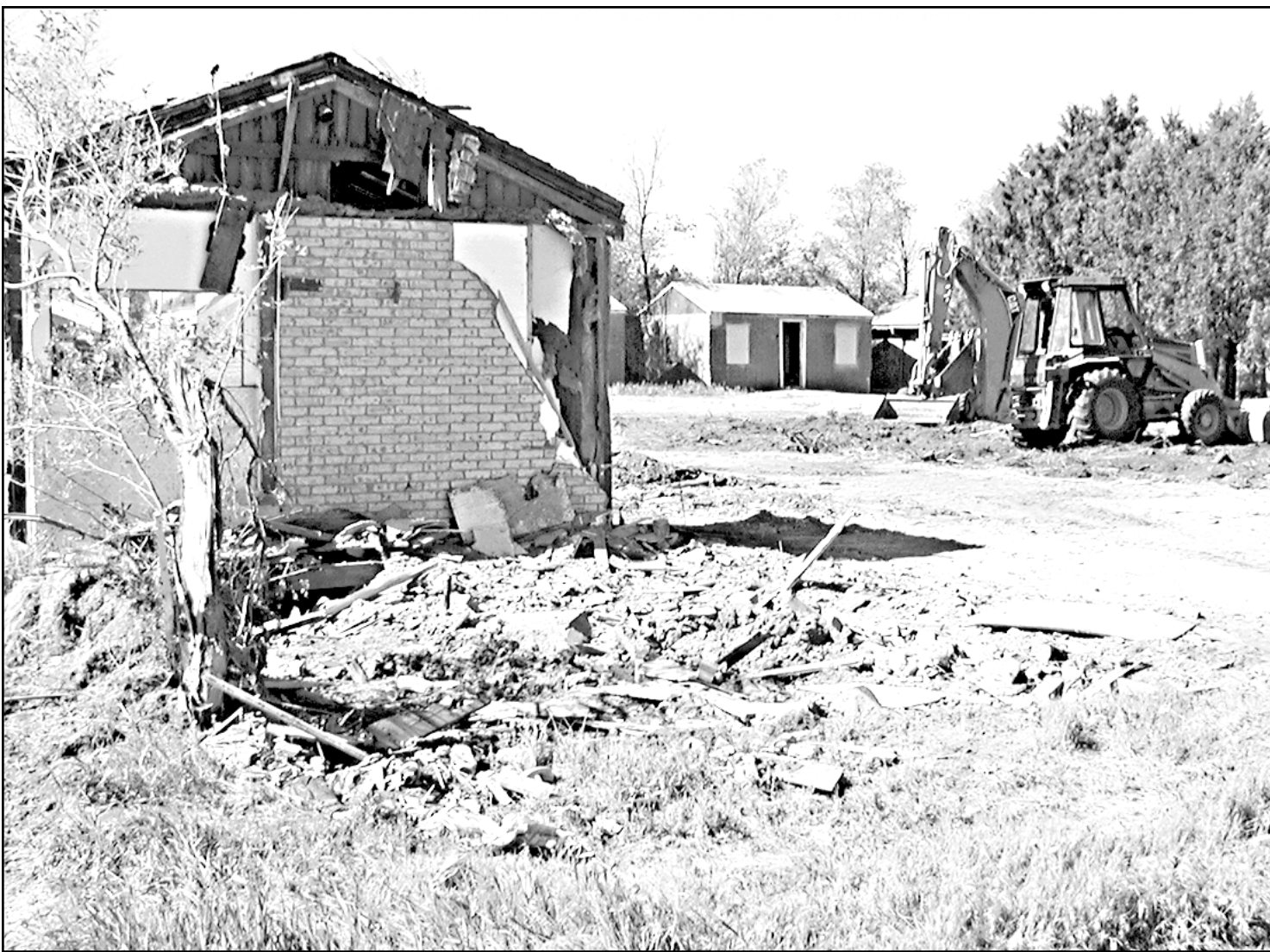
Goody's, owned by Mike Yarger, began demolition of the K-Inn at Business U.S. 24 and Cherry last week. City Building Inspector Steve Criswell said it appeared about a third of the motel had
