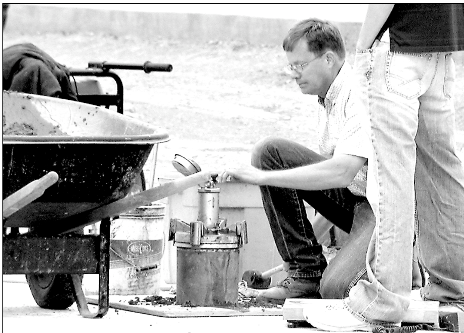
Jerry Nemechek of Evans, Bierly, Hutchison and Associates tested cement being poured for a section of 17th Street at Broadway Tuesday morning. The south half of 17th should be open shortly after
