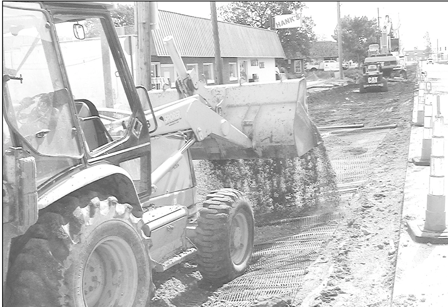
Traffic on 17th Street is still one-way, but from the railroad tracks to Main, now drivers are on the new concrete south half of the street. Workers switched the side of the street on Monday, and by Wednesday they had removed old bricks all the way to Caldwell. Workers were laying the rebar matting and leveling the base in front of Hank's Café to get this section
