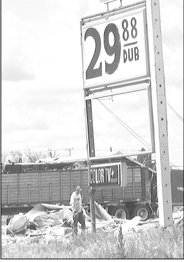
More than 80 percent of the old K-Inn motel is gone, and the last pieces are expected to be removed in the next few days. The old motel on Business U.S. 24 near the Cherry intersection, was ordered demolished after more than a two-year court fight. The city is paying Goody's, owned by Mike Yarger, to remove the buildings.
