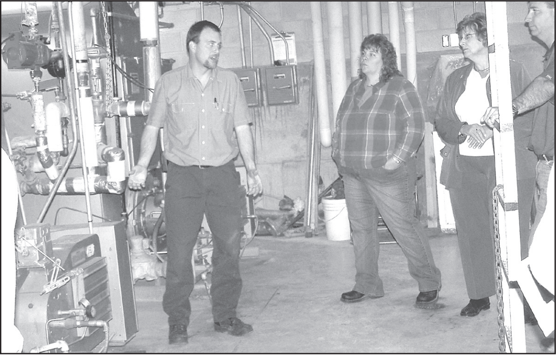
Neil Normandin, maintenance director at Goodland Regional Medical Center, gave hospital board members a tour of recent updates made to the physical plant. Board members, from left, are Mary Volk, Joyce Moore and Darin Neufeld. Photo by Tina Goodwin/Goodland Regional Medical Center
