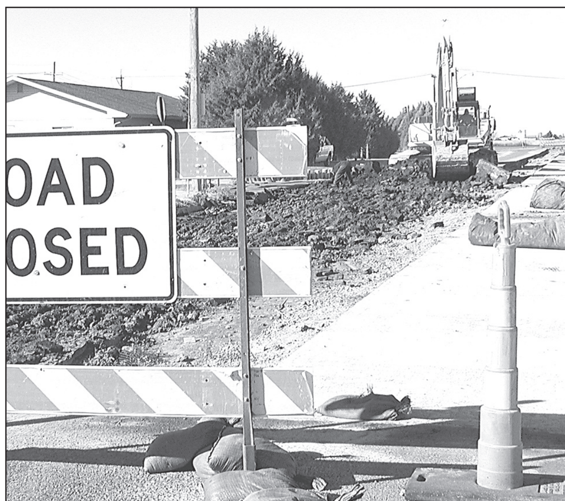
Crew workers from Oakley-based Sporer Land Development, Inc. prepared the south side of 8th Street Wednesday to lay down fresh concrete. The street is closed from D'Lao to K-27. Photo by Ramona C. Sanders/The Goodland Star-News
