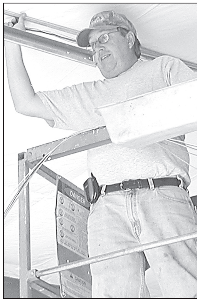
Marty Johnson, owner of Marty's Electric, worked on the wiring in the expansion at Herl Chevrolet Buick the last week of October. Owner Jay Herl said the business will probably be using the new addition by January.
