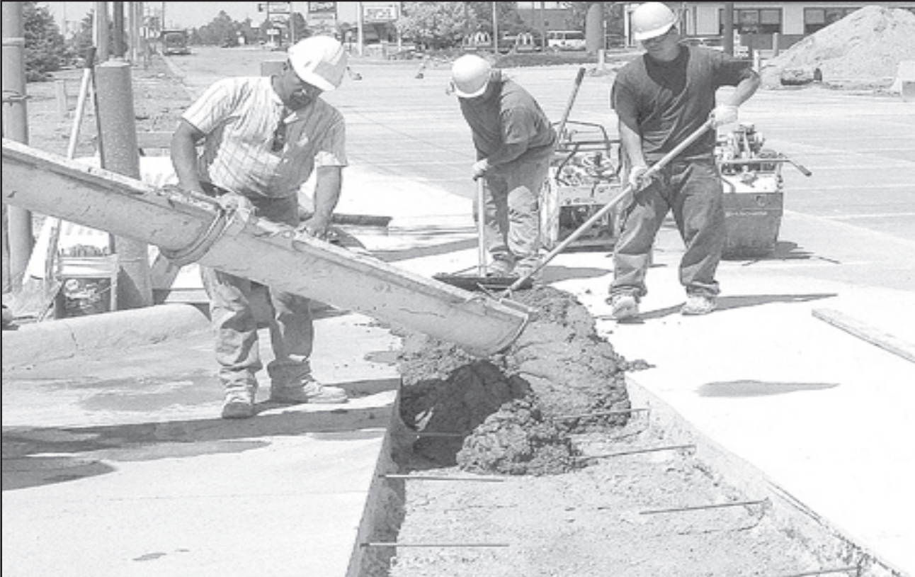
Workers from Miller Construction poured the final piece of the new section of Enterprise Road that runs from McDonald's to the intersection at 25th Street in front of the Conoco Travel Shoppe, owned by Service Oil. The street should be open by the middle of next week, said Rich Simon, city public work director. Miller is ready to
