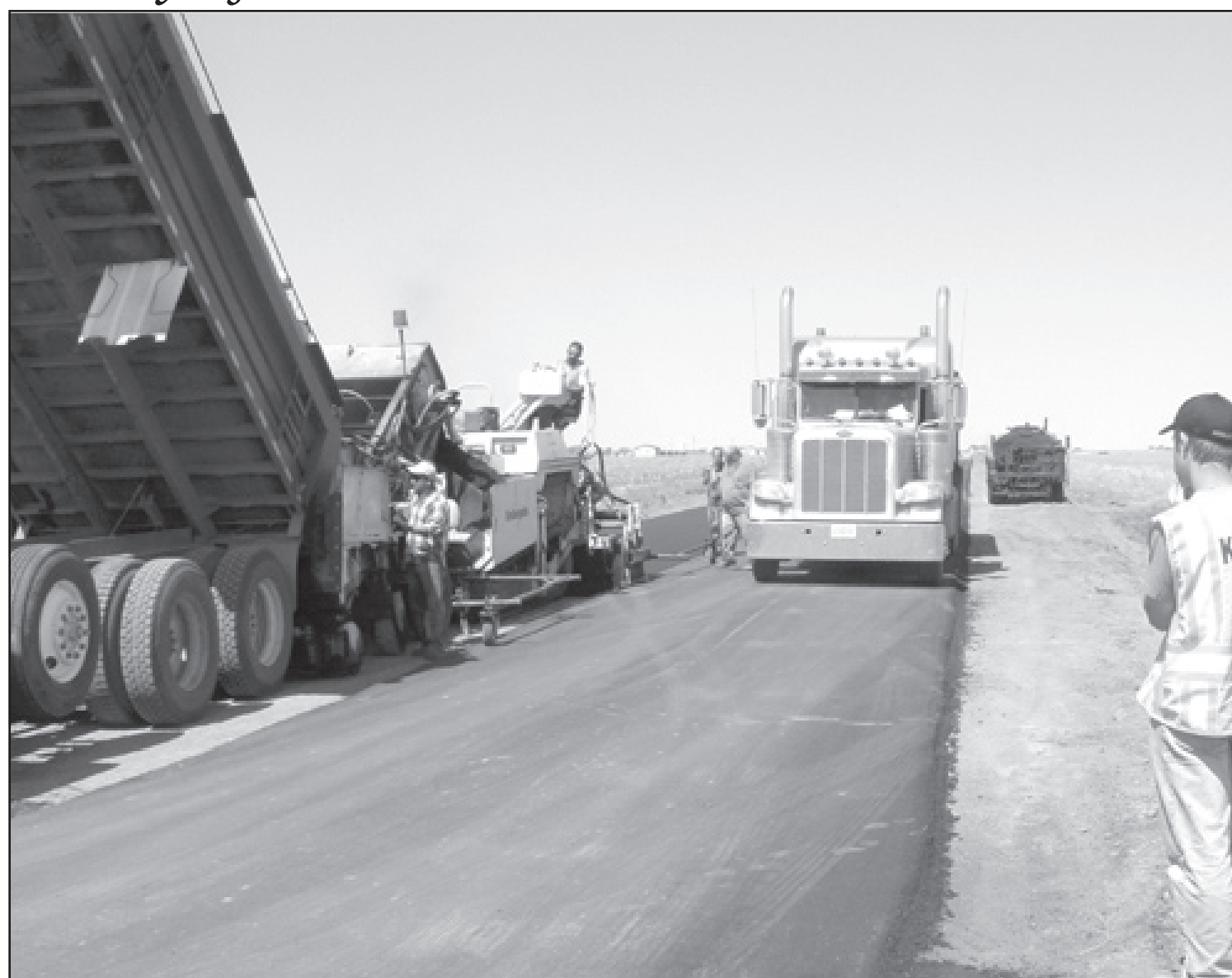
The first layer of asphalt went down on County Road 65 (West Eighth Street) Saturday morning, when a crew from Venture Paving of Great Bend reached K-27. Brad Geist (right) was keeping track of the loads of asphalt. The crew planned to turn around and start the second lift. Paving a five-mile section from K-27 to
