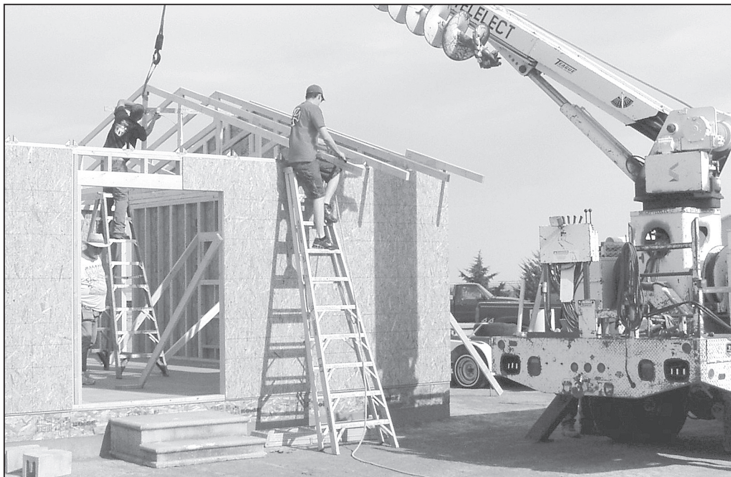
Darrell Hoss (center, on the floor) and son-in-law Chris Dorn (right) get help from T.J. Yarger (left) on an addition to the Total Look, 691 E. 25th St., to house a shower, laundry and extra space for Deedi Hoss-Dorn's facial services. Helping, but not in the picture, were Darrell's son Clayton and Mike Yarger, who operated the crane. Photo by Jordie Mann/The Goodland Star-News
