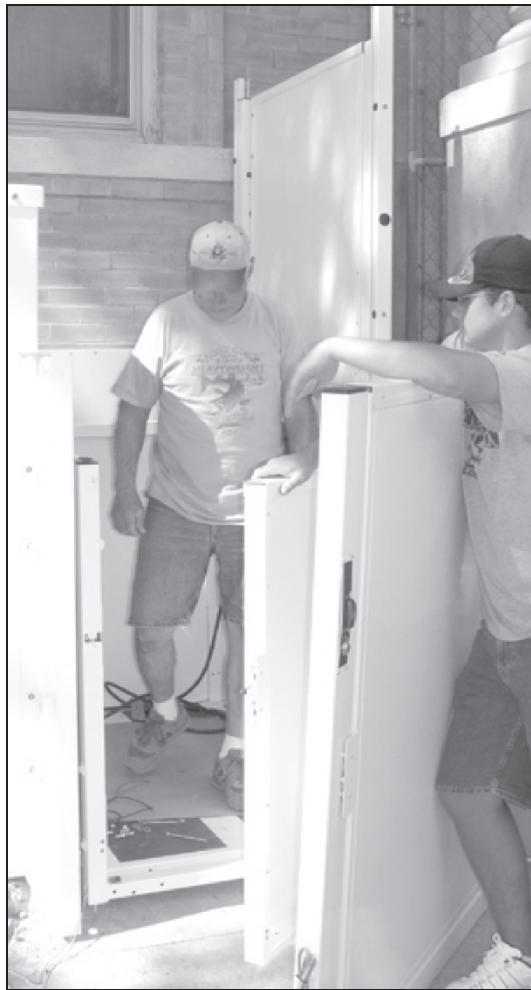
Albert Burton (inside lift) and his son Caleb, from Hill City, installed the new outdoor handicapped lift at the Carnegie Arts Center last Tuesday, but at the end, Burton found a small part was missing. Photo by Tom Betz/The Goodland Star-News
