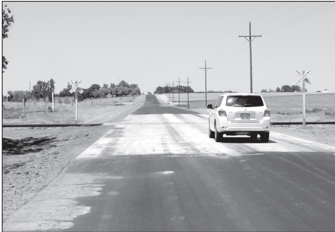
A car crossed the new concrete railroad crossing Wednesday morning on County Road 16 south of the Sugar Hills Golf Course. Paving Road 16 is one of the last pieces of the city, county joint road projects. The new paved road was one of the projects approved by Sherman County voters two year ago.
