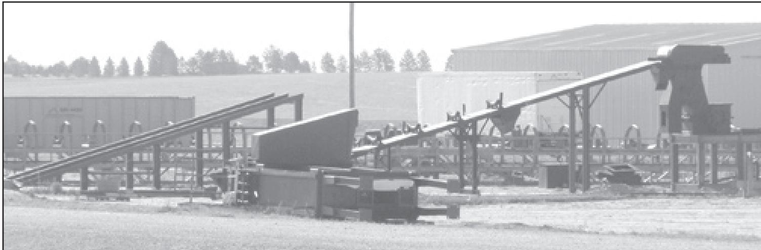
Sections of the fuel delivery system lay on the ground at the site of the Goodland Energy Resources coal-fired power plant being built five miles west of town. The potential purchase of the plant by Energy Holdings Ltd. has halted work at the site.
