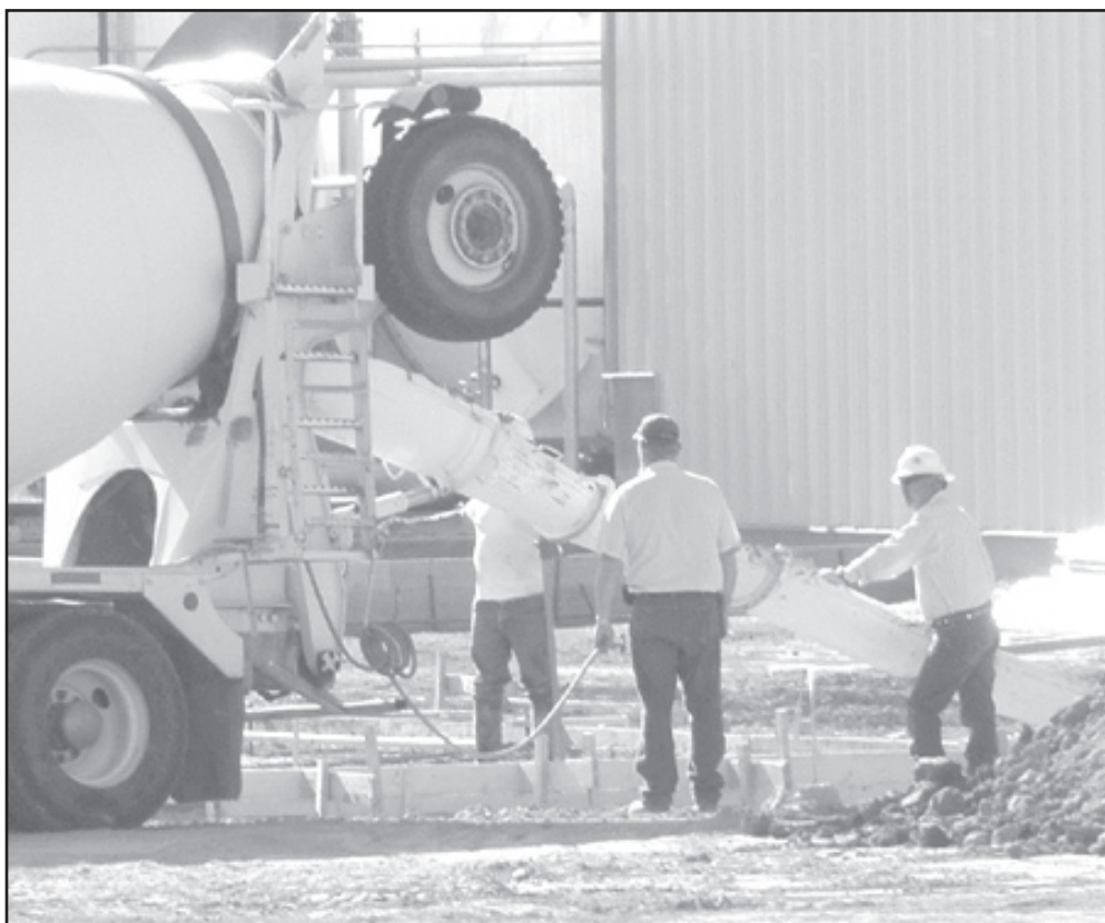
A crew helped pour concrete for a pad for ancillary equipment at the E-Caruso Ethanol Plant being built at the Goodland Energy Center five miles west of town. The plant is getting closer to being ready for testing and operation. Photo by Tom Betz/The Goodland Star-News
