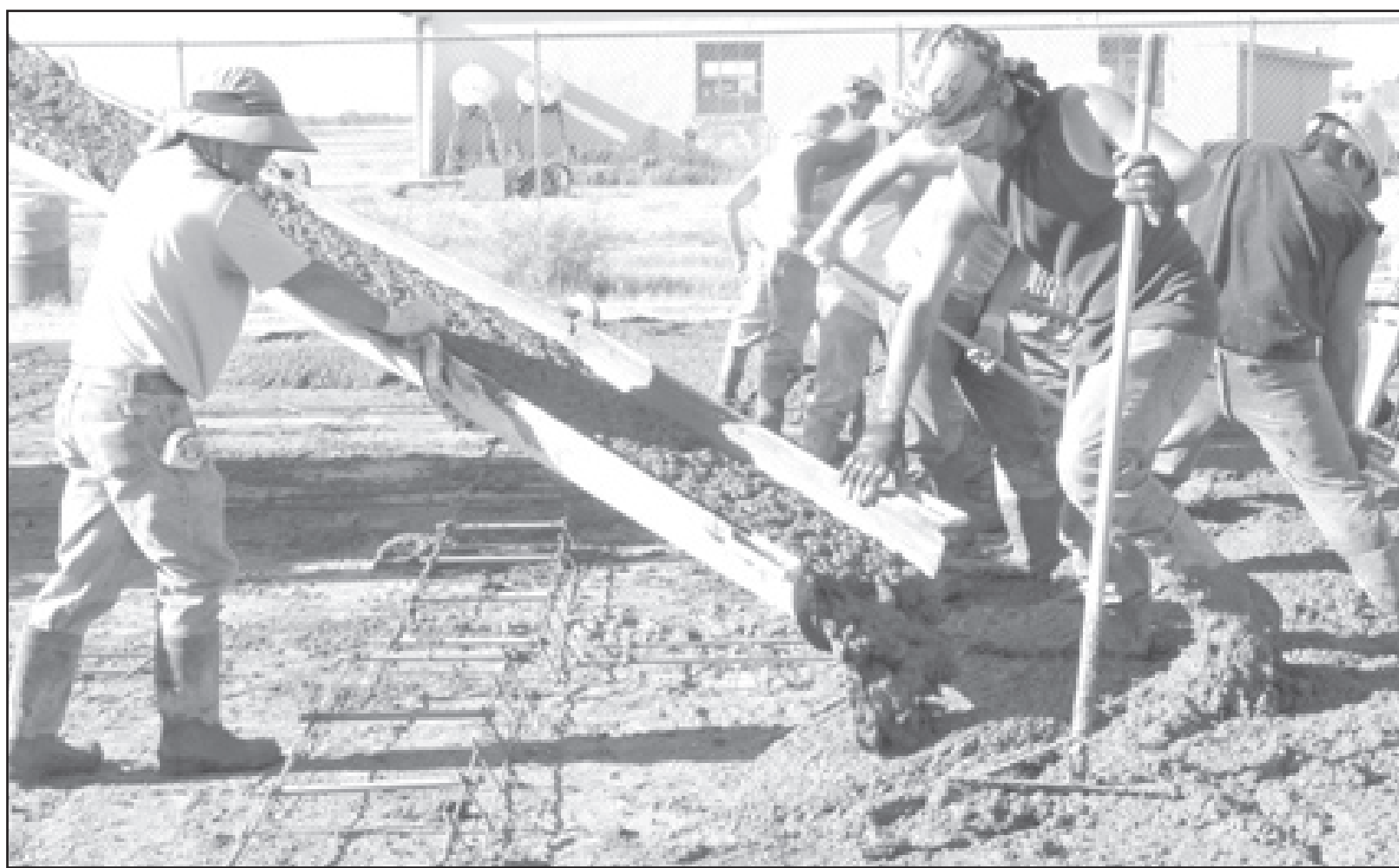
Mike Miller, owner of Miller's Construction directed a stream of concrete as his crew worked Tuesday morning, pouring and smoothing the new entrance to Renner Field. The $521,720 project is being paid with a $286,000 grant from the Federal Aviation Administration and the rest from the city.
