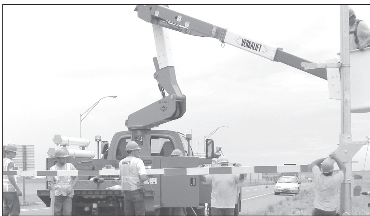
State highway employees installed a snow gate on I-70 west of Goodland as part of a program to improve road safety during winter blizzards when the highway has to be closed down.
