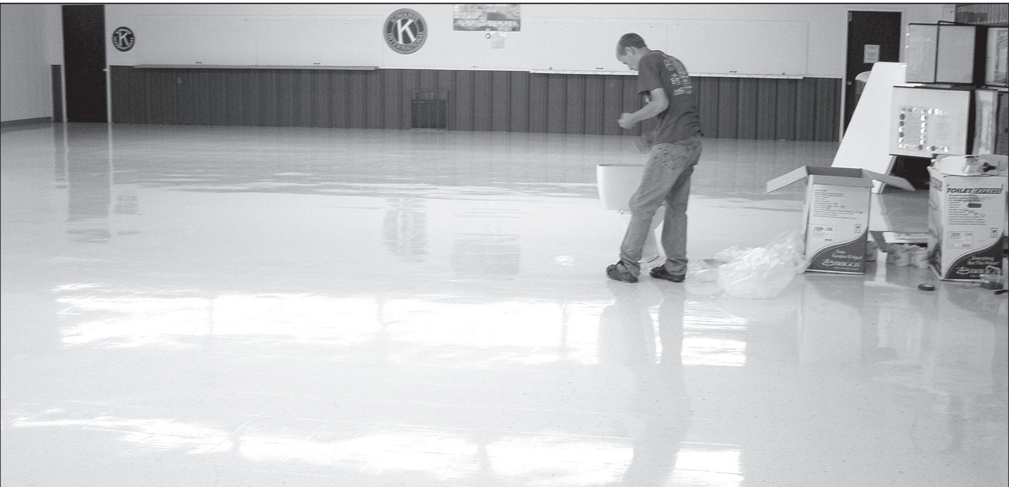
Adam Duell checked the fittings for a new toilet that was installed in the men's restroom at the 4-H building on the Sherman County fairgrounds. The toilets were sitting on paper on the newly replaced and waxed floor, which was completed last week. The restrooms got
