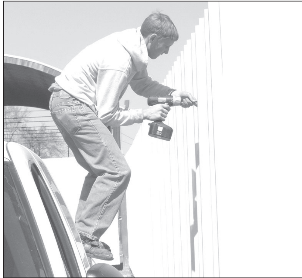
Adam Duell, son of Steve Duell, chairman of the county Fair Board, used a battery-powered drill to put screws in the top part of a new steel sheet fence in March on the south end of the Sherman County Fairgrounds which separates the race track and arena from the carnival. Steve Duell was marking the line of screws with the help of farmers Scott Jarrett and Art Hatfield.
