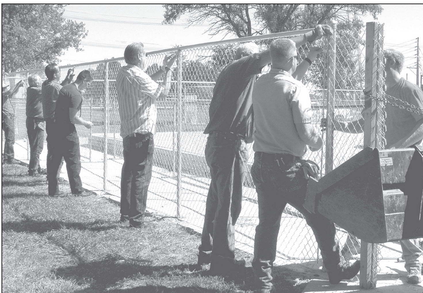
City employees helped erect the chain link fence around the Skate Park on Wednesday afternoon. Helping were (l to r) power plant employees Bill Bowen, Kendall Gittinger, Roy Wassemiller, Fire Chief Brian James, Building Inspector Steve Criswell,
