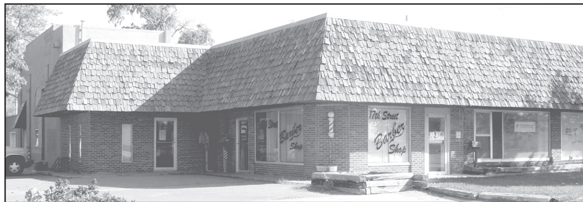
Sherman County now owns the building at 212 E. 17th, which they accepted as as donation from Walt Adams. The Sherman County Economic Development Council will manage the property, and the county will help pay to fix the roof. Photo by Tom Betz/The Goodland Star-News
