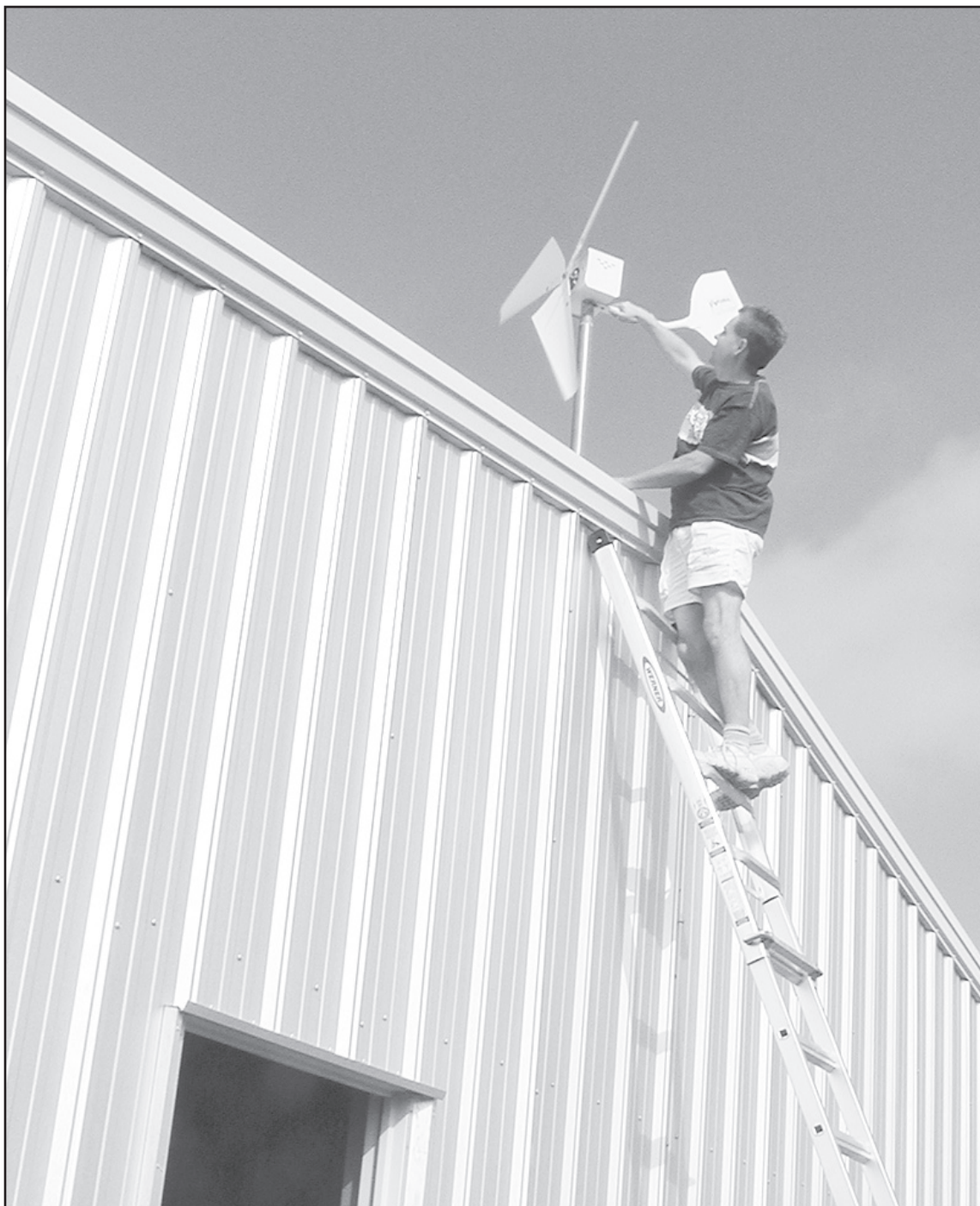
Marlin Queen climbed the ladder to adjust the wind turbine on the building at Reeser's home near St. Francis. He, along with Ron Wieck and Tanner and Ben Lacy installed the wind power equipment. Photo by Karen Krien/The St. Francis Herald
