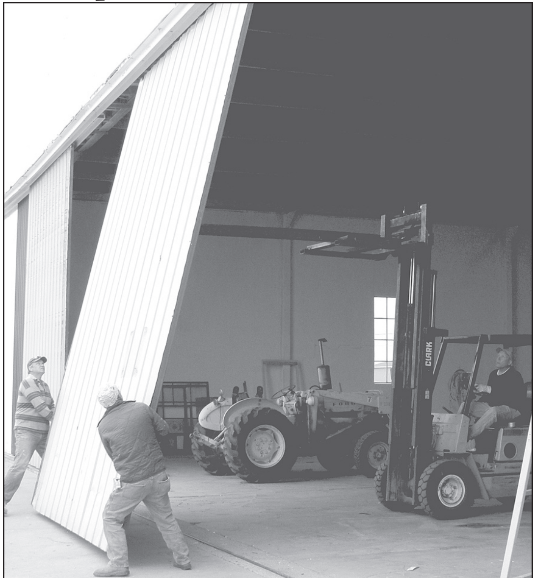
Resurfacing the hangar doors is the last step in rehabilitating the old 1934 WPA hangar at the Goodland airport. Saturday Dean Oharah (left) Frank Black (center) and John Topliff (left on lift) removed the last of the old hangar doors and Oharah and Black put new bronze aluminum sheeting on the doors and got the wheels loosened up. Topliff said this step completes this phase and he plans to add the addition to the east side next summer. Photo by Tom Betz/The Goodland Star-News
