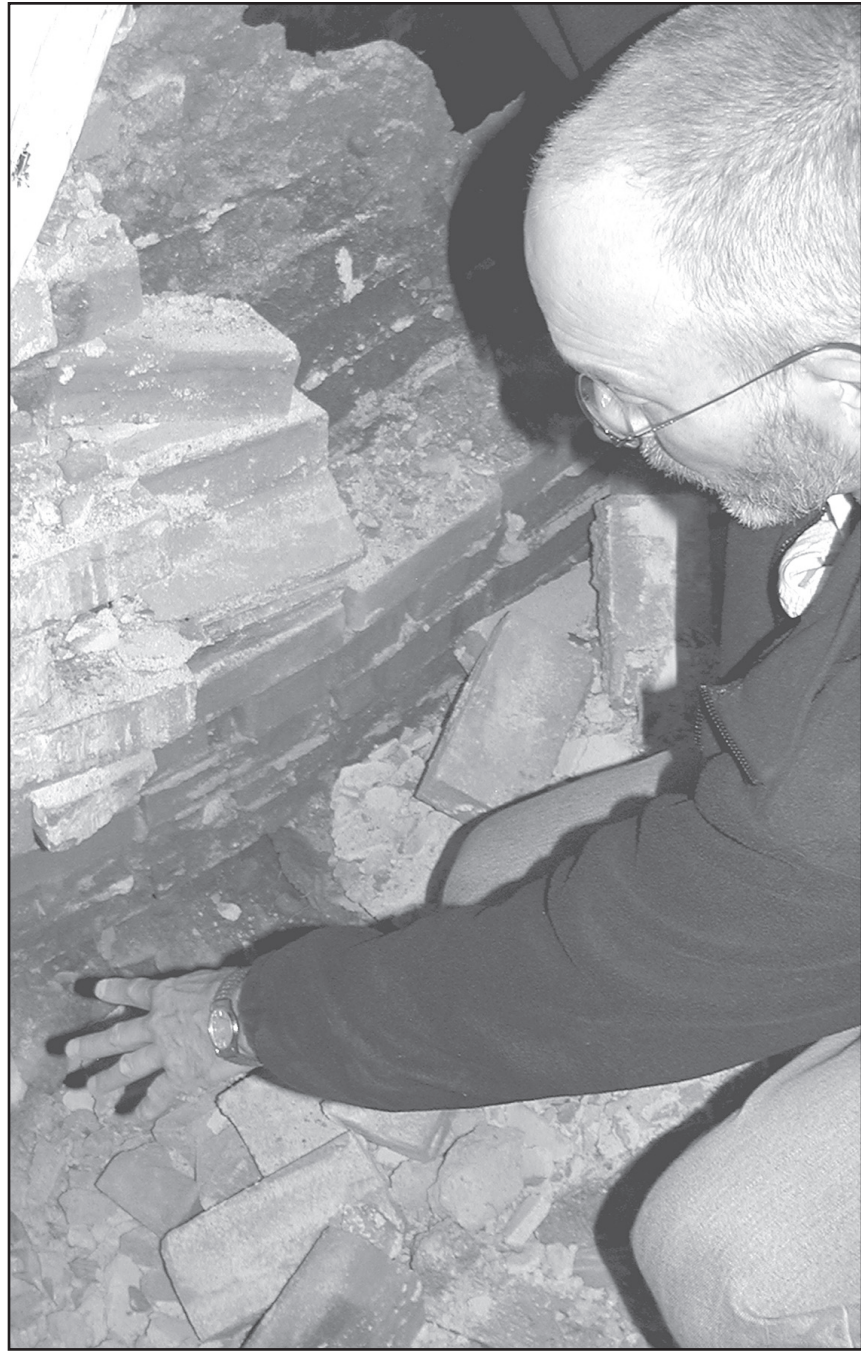
David Branda, Sherman County Historical Society president, pointed out where bricks had fallen and crumbled mortar piled up at the base of a wall in the basement of the Ennis-Handy House that buckled when work was being done on the sewer. Despite the need for repairs, the house is decorated for Christmas and is available for holiday parties. A 12-foot tree, donated by Wal-Mart, was cut to fit under a 10-foot ceiling in the front room of the house and decorated by board member Christie Rasure.
