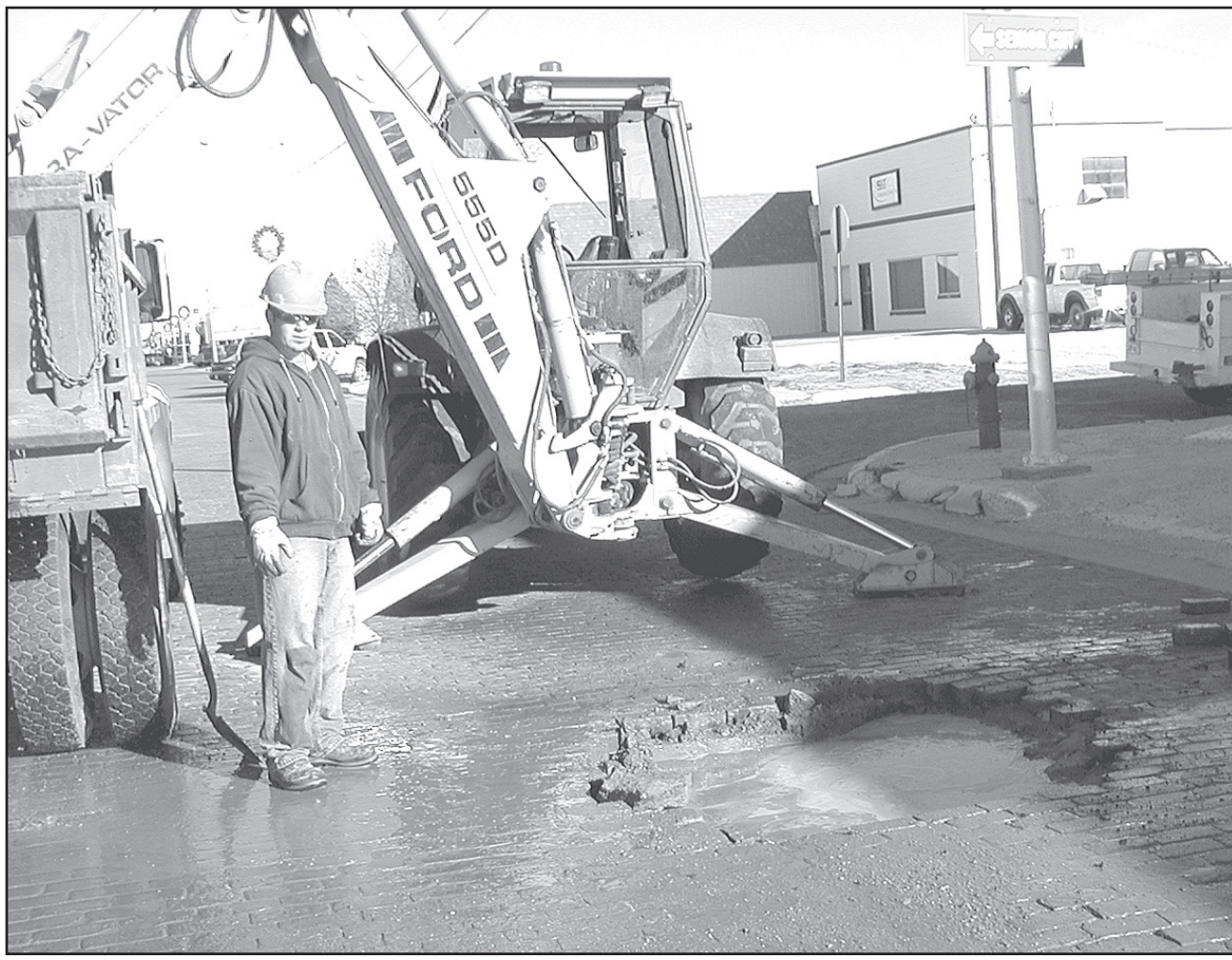
City of Goodland employee Mike Reyes worked on a water leak at 1507 Main. Water filled the hole and was running down the street. Reyes thought the leak probably started Sunday night.
