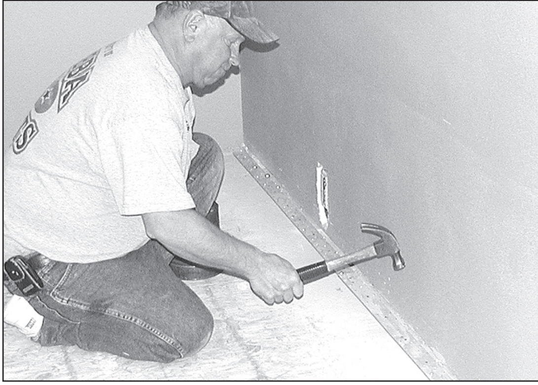
Bob Rohr was putting down tack strip in preparation to lay carpet at the First Baptist Church's new location at the former Alco store on Main Avenue. The church hopes to be holding services there in the near future. Photo by Pat Schiefen/The Goodland Star-News
