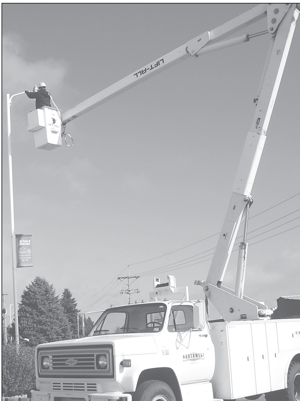
Students in the electrical department of Northwest Kansas Technical College worked with a bucket truck donated by Midwest Energy to the department. Safety equipment and inspection of the truck were also donated.
