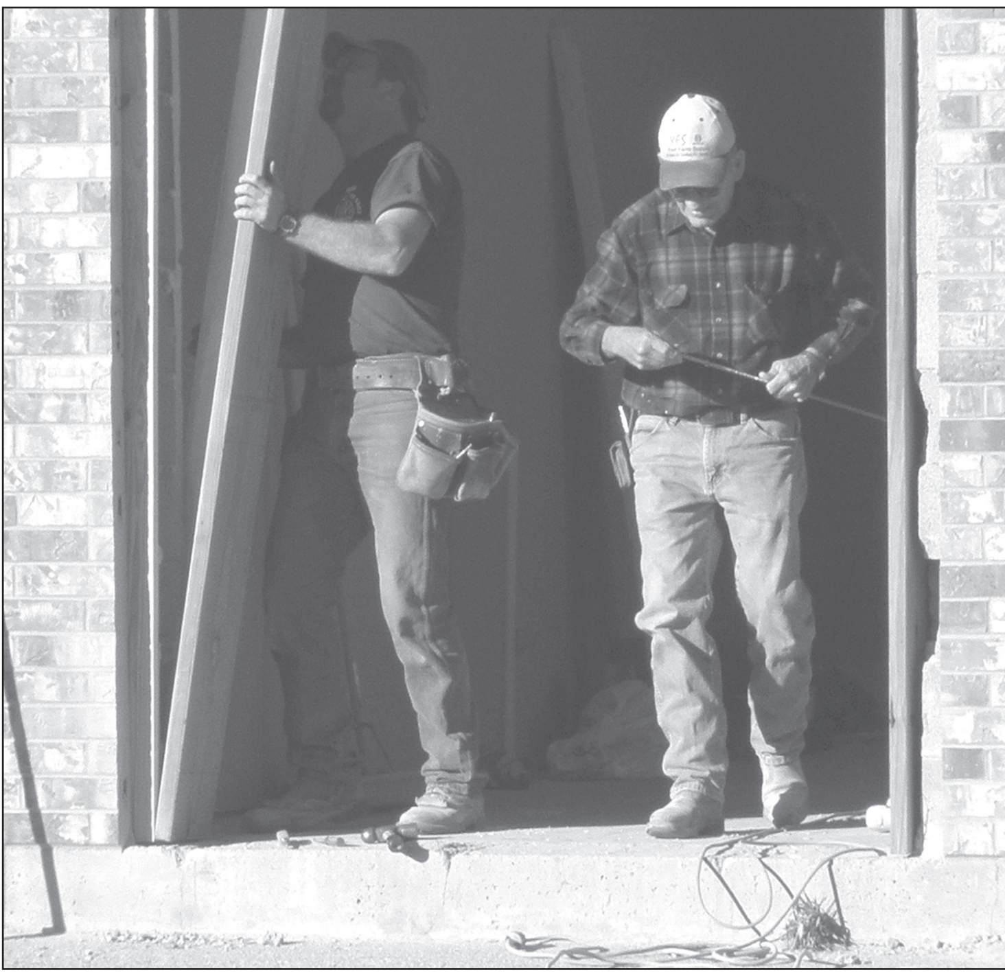
Ralph Brighton (left) and Darrel Schrader (right) framed out a new side door installed in the wall on the south side of the First Baptist Church on the corner of Main Ave. and 12th Street. Schrader said the church is moving forward and working on finishing the inside installing carpet and tiles.
