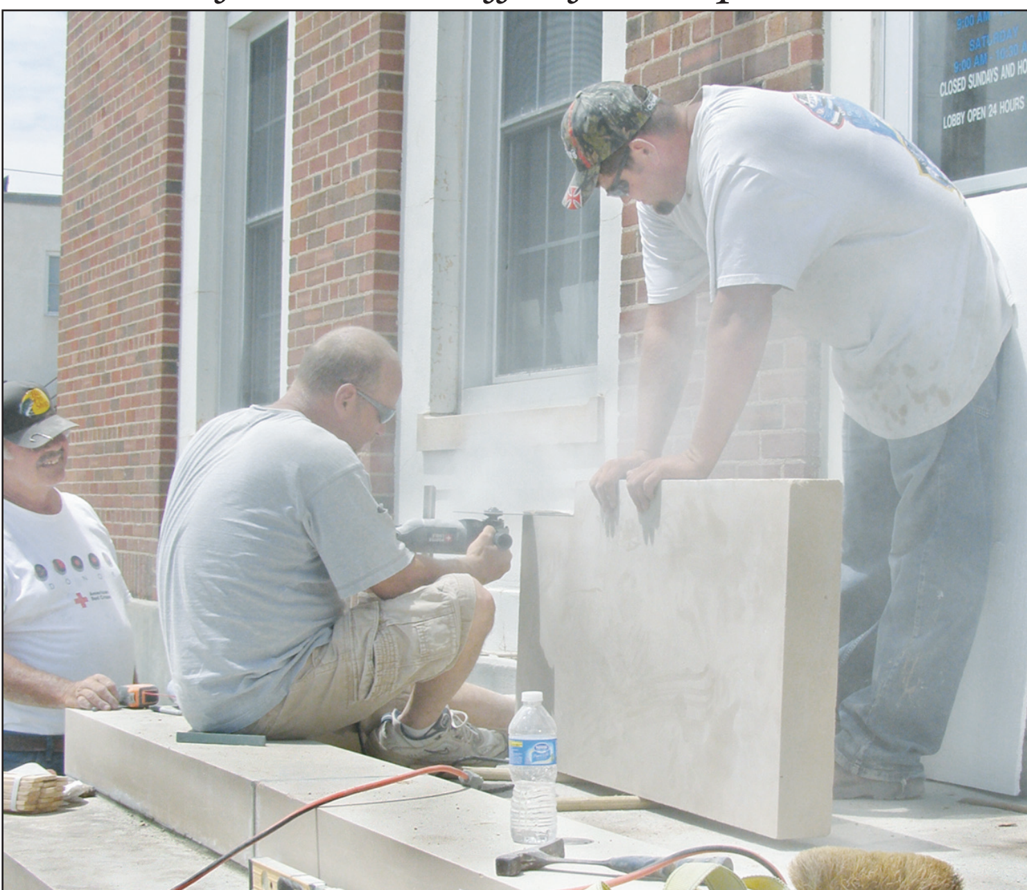
Several weeks ago a company came to town to replace the front steps at the Goodland Post Office, and last week a company from Fort Scott came to put pre-cast stones on top to finish out the new steps. The front steps are expected to be open this week. Photo by Tom Betz/The Goodland Star-News
