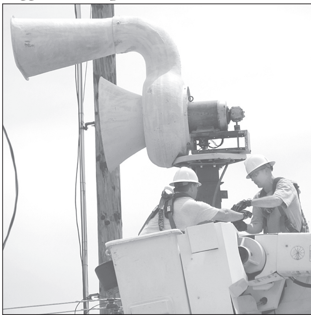
Workers from the City of Goodland worked on the sirens behind the City Building, 204 W. 11th. The sirens are used for fires and tornado warnings.
