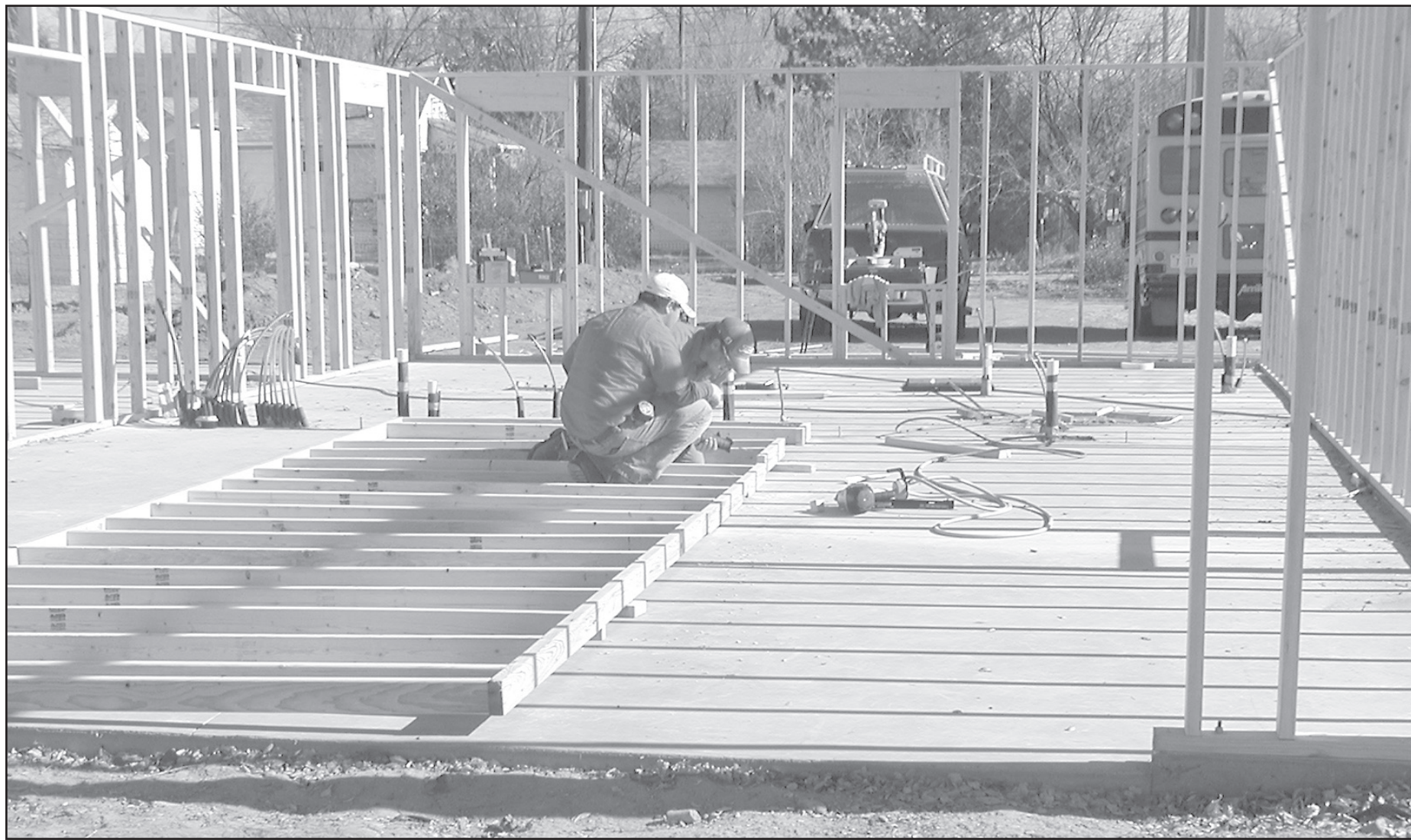
Northwest Technical College carpentry students work on the latest building project for the school. Getting to work on an actual construction gives the college's students real world experience. The project is located across the street east from
