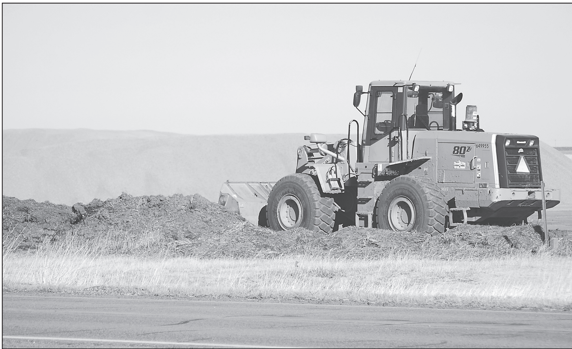
The Kansas Department of Transportation has cleared a patch of land at the Brewster I-70 exit and begun staging material there for summer road projects. Photo by Kevin Bottrell/The Goodland Star-News
