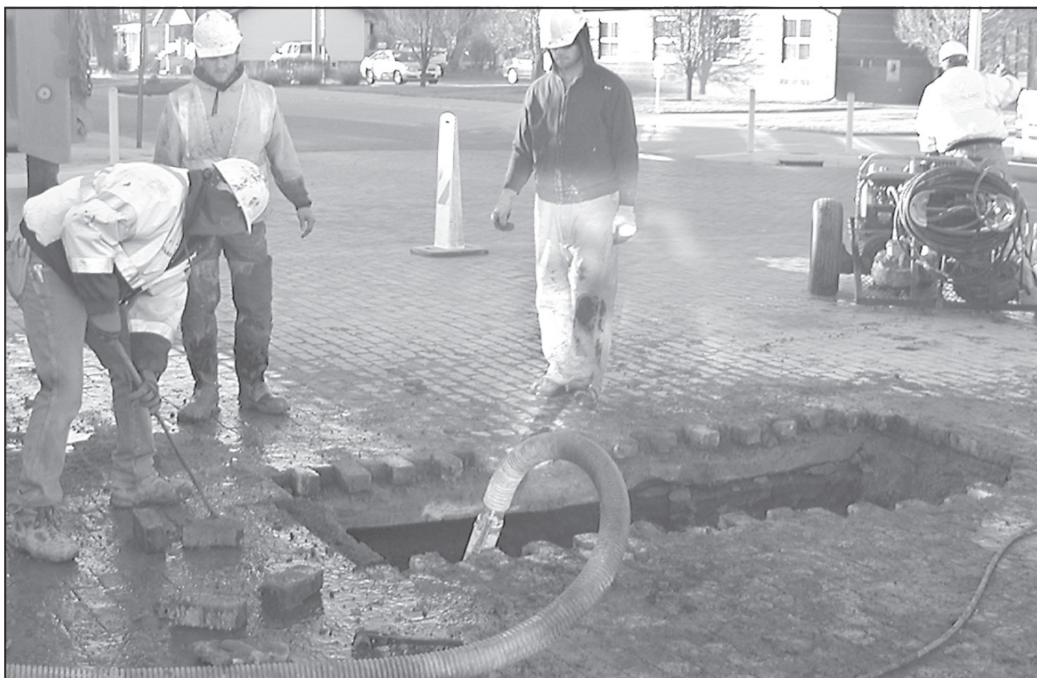
It was a bitter cold day earlier this month when city crews had to begin repairs on a water line on Main Street near Central Elementary. The line has now been fixed and the bricks replaced. Photo by Kevin Bottrell/The Goodland Star-News
