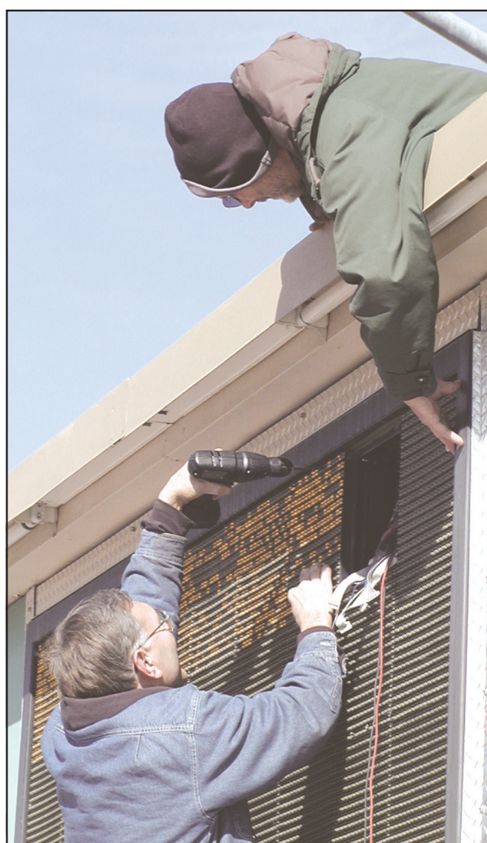
Sherman Theater owner David Branda and Randall Fixsen with Fixsen Electronics worked on the theater marquee Friday afternoon. The marquee had one panel that wasn't working. Photo by Kevin Bottrell/The Goodland Star-News
