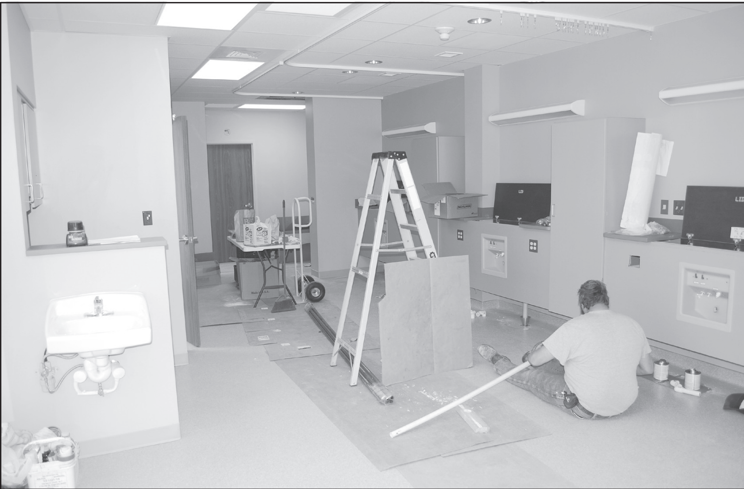
A workman was installing the water hookups for the dialysis unit at Goodland Regional Medical Center in early February. The hospital hopes to have the unit up and running by April 1. – Photo by Kevin Bottrell/The Goodland Star-News
