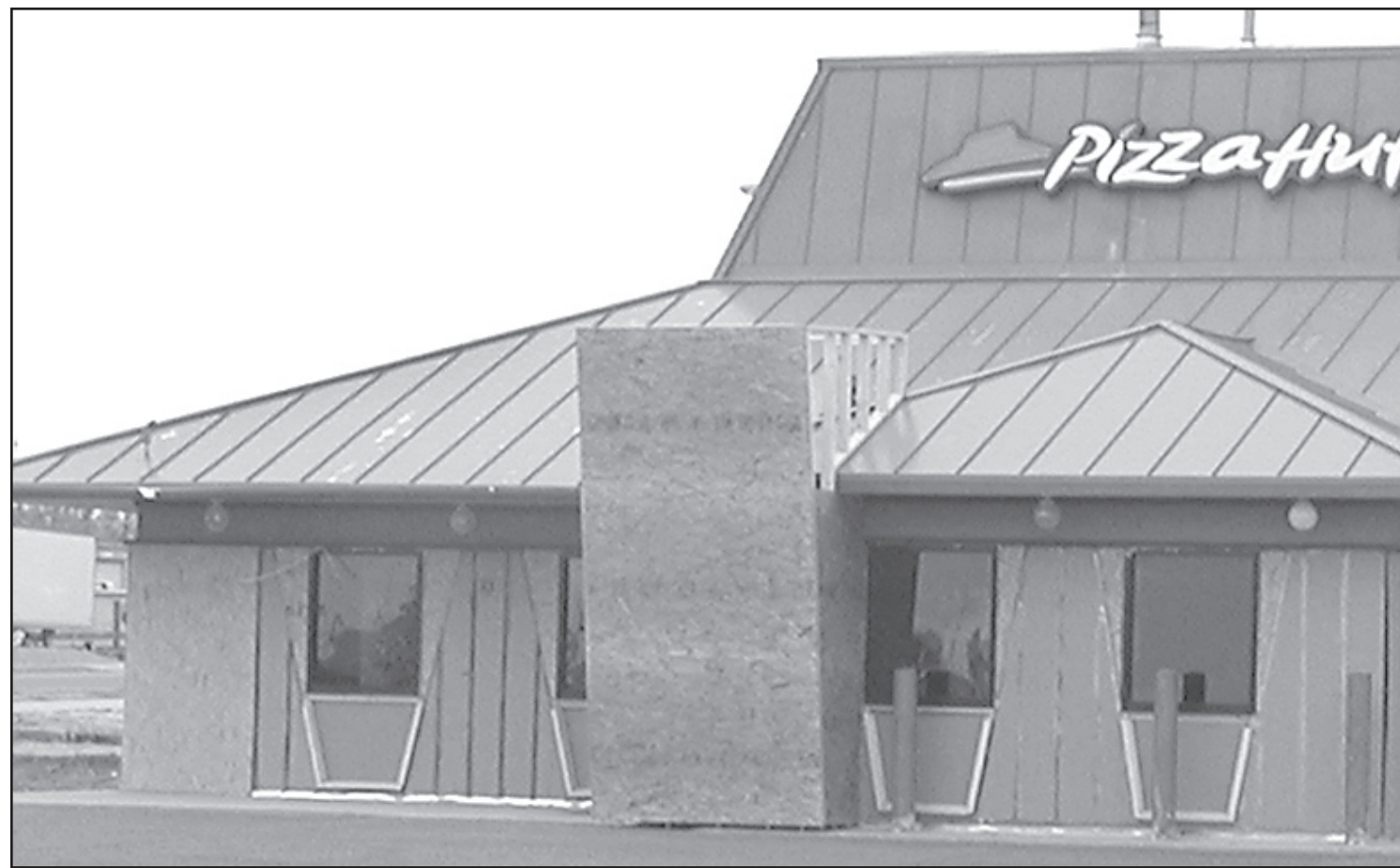
The Goodland Pizza Hut is having work done on its exterior. Last week one entrance was closed off while it was being worked on. The restaurant is also having landscape work done. Photo by Kevin Bottrell/The Goodland Star-News
