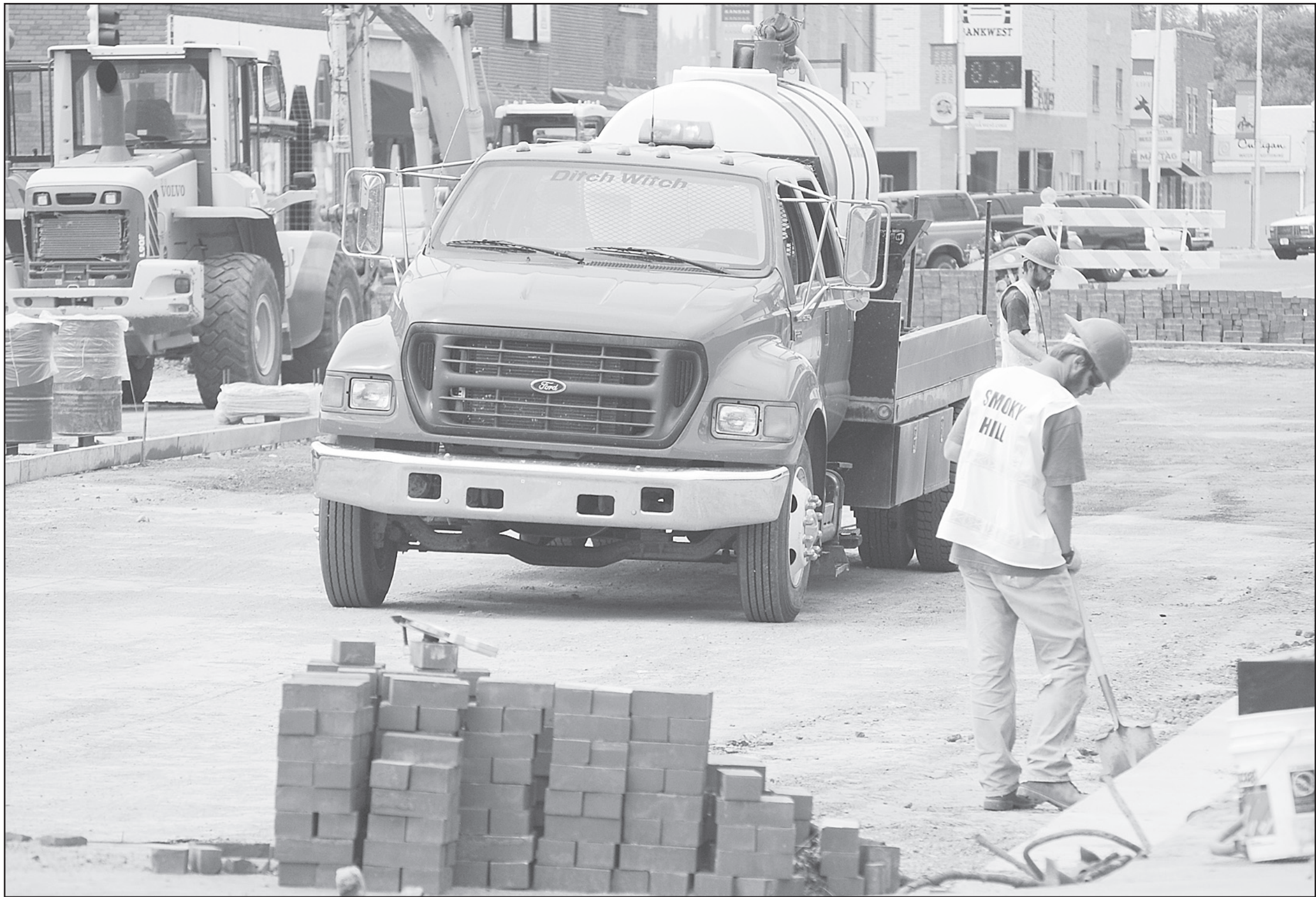
Construction crews were preparing the Main Avenue construction site for concrete pouring this week. The workers have already hooked up the new water pipes running under the sidewalk, and once the concrete on the street has set, another company will come in to lay the new brick. The contractor told the Goodland City Commission on Monday that the project is on schedule. Photo by Kevin Bottrell/The Goodland Star-News
