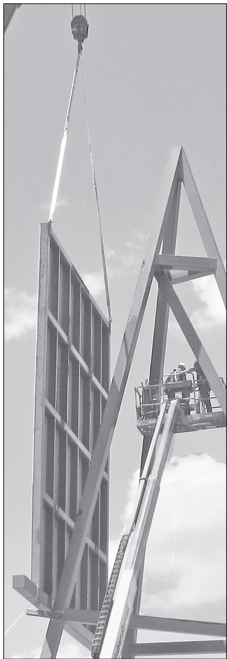
Once the welds were cut and the painting was detached, a crane was used to lower it to the ground.
