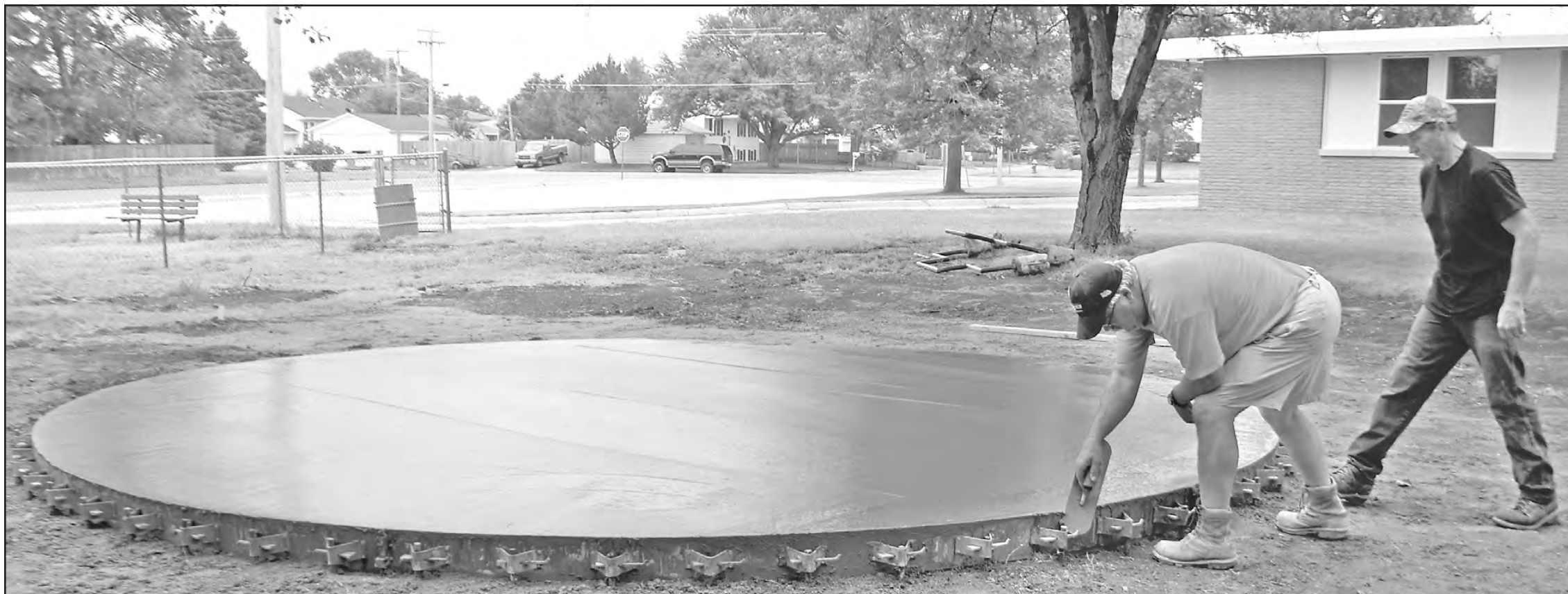
The First Christian Church, 811 Arcade, is in the process of building a labyrinth north of the main building. They started construction on the project on Wednesday. After the concrete is poured a seven circuit labyrinth will be painted on it. Highway paint will be used and then it will be sealed.
