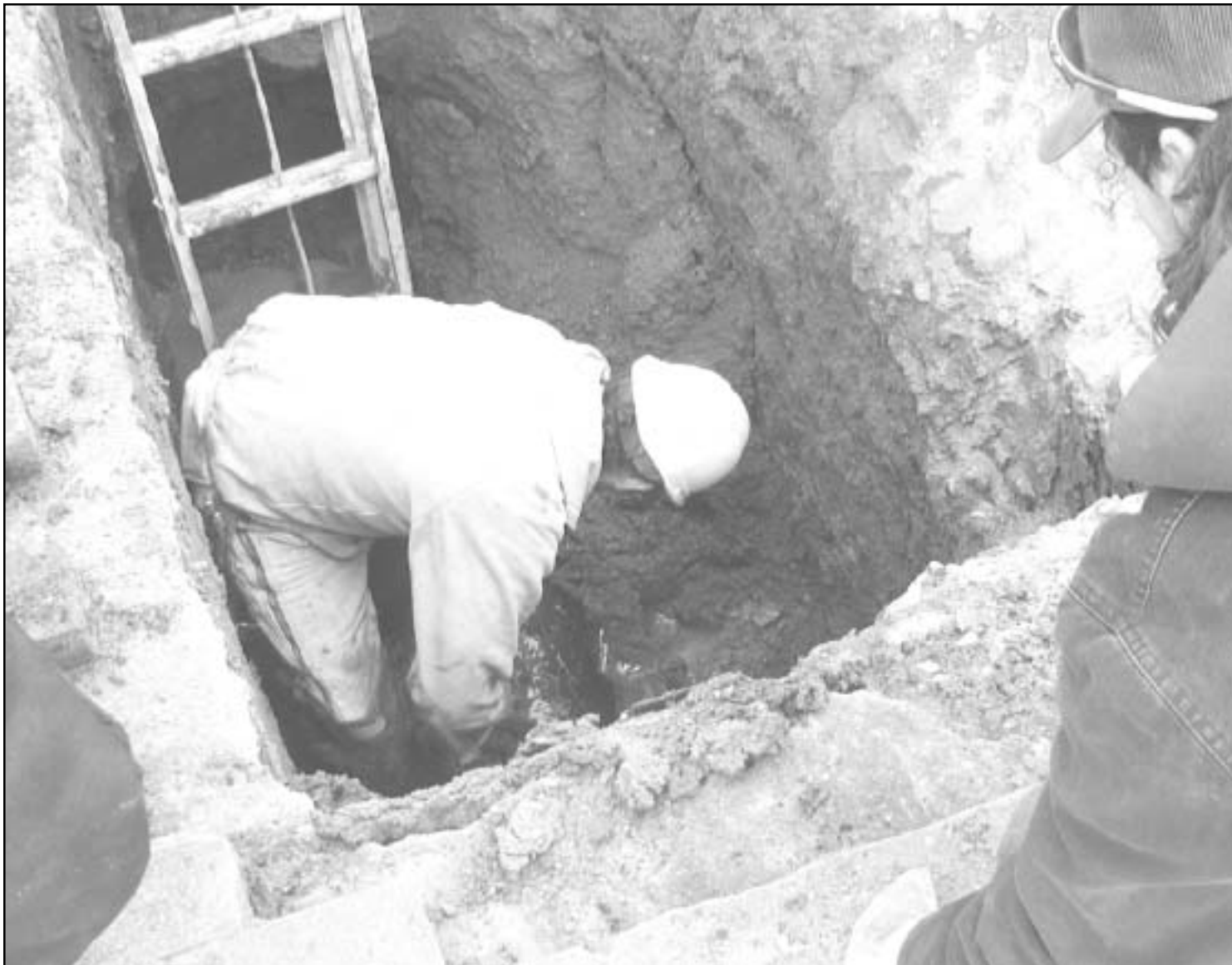
Joey Snethen of the city's water department looked for water leaks as a co-worker watch for cave-ins Tuesday morning under 17th Street, between Clark and Broadway Avenues. Two separate leaks were found and repaired.
